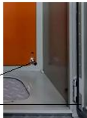
Studs Provided In The Box as Well as on The Door for Protective Earthing
